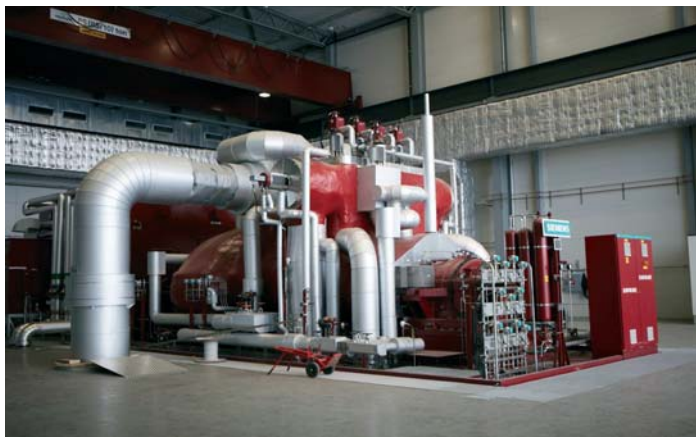
The generator and the turbine. The turbine is one of the largest ever built by Siemens for a bio-fuelled plant.
